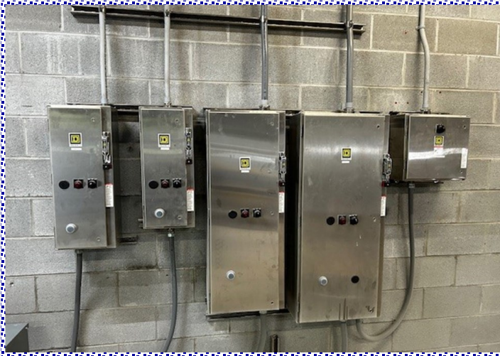
Completed control Panels at Splash Island, PICP
