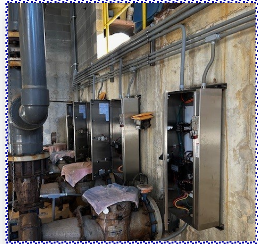
Completed control Panels Whirlin' Waters, WCP
