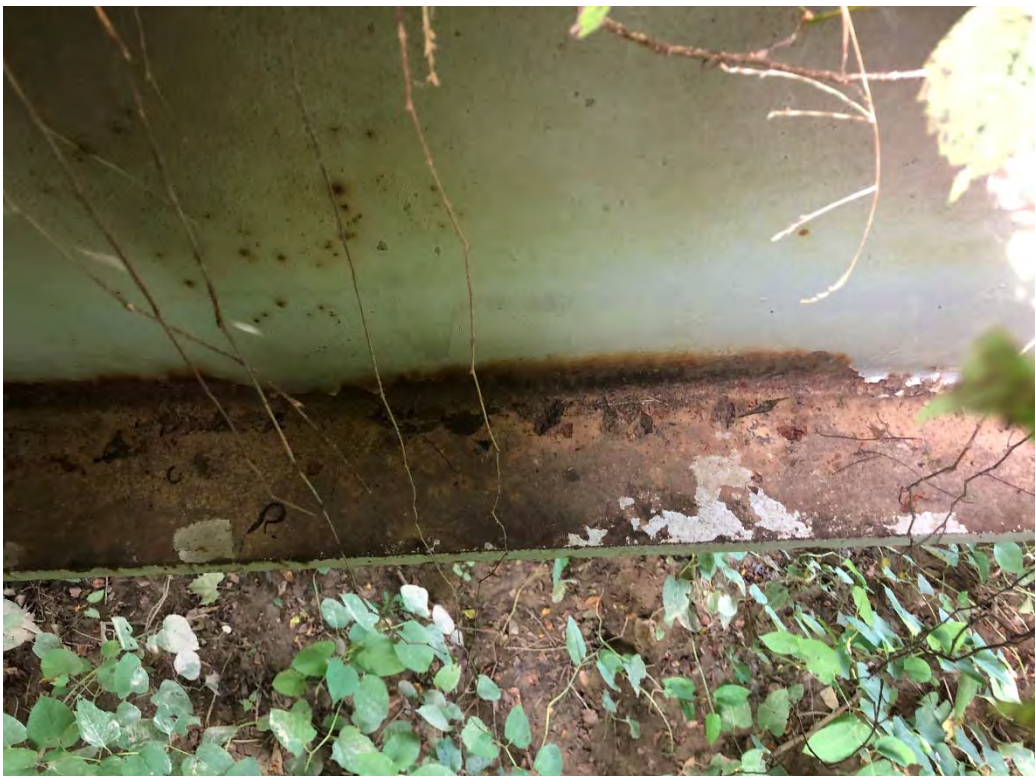
Typical light rusting of beams.
