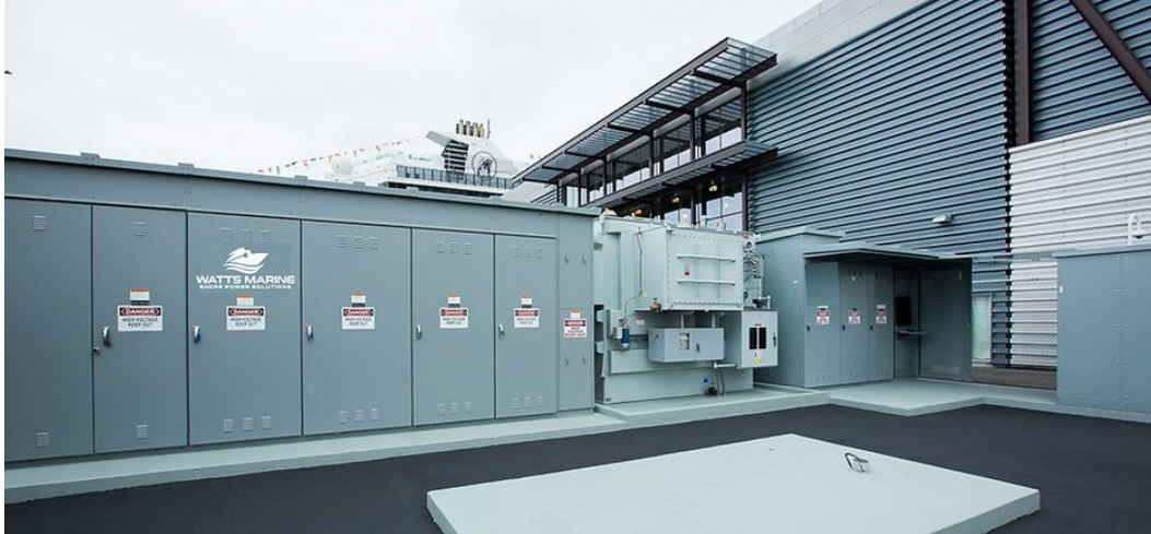
Figure 2-4. Dock Mounted Shore Power
